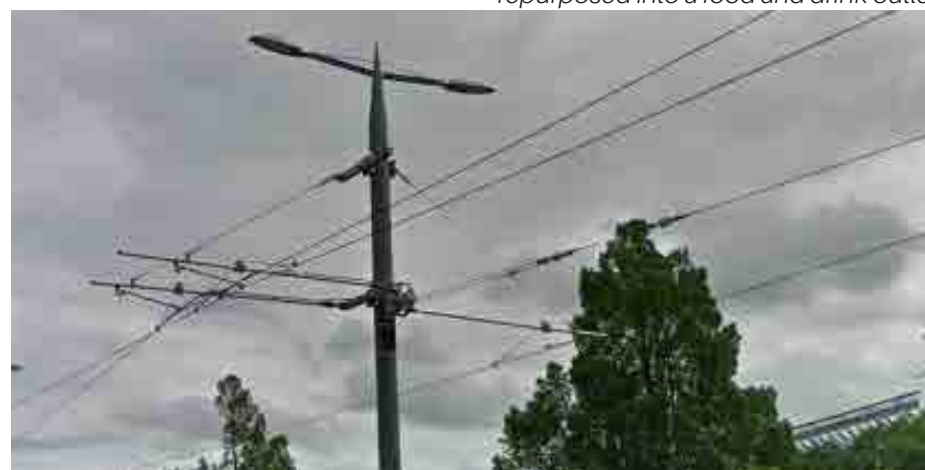
Figure 6.139 Modern tramline pole with high level wires and integrated street lighting.
