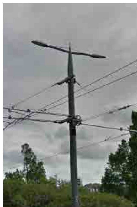
Figure 5.27 Modern tramline pole with high level wires and integrated street lighting.
