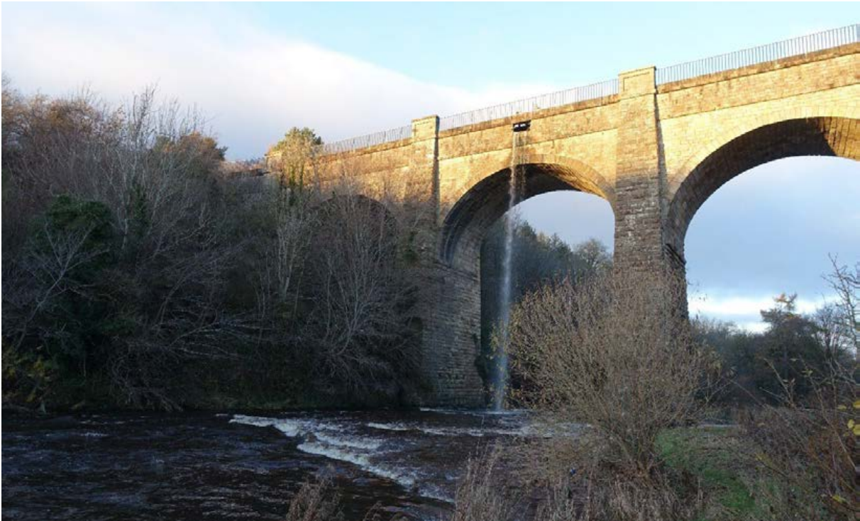
Figure 3.24: Lin's Mill Aqueduct passing over rapids in the River Almond, a sluice allows excess water to fall from the canal into the river below
