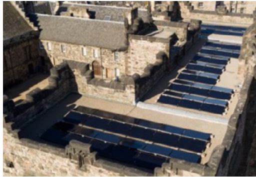
Solar panels hidden behind parapet at Edinburgh Castle ©Historic Environment Scotland
