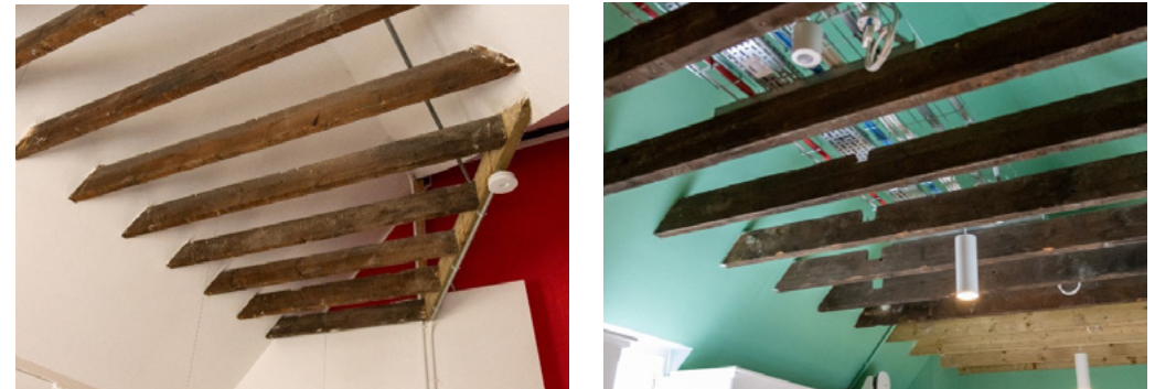
Surface mounted services behind original roof beams.
