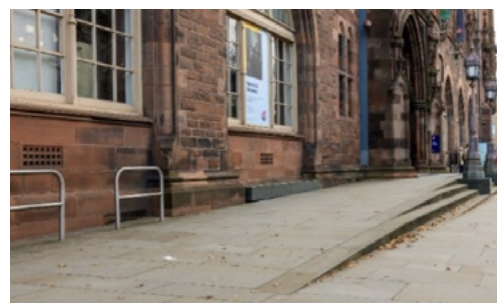
Regrading of ground to achieve level entrance at National Portrait Gallery, Category A listed, LB27764, 14/12/1970.
