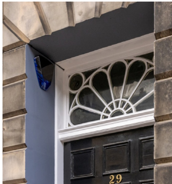
Good example of a sensitively positioned security alarm box on ingoie of doorway.
