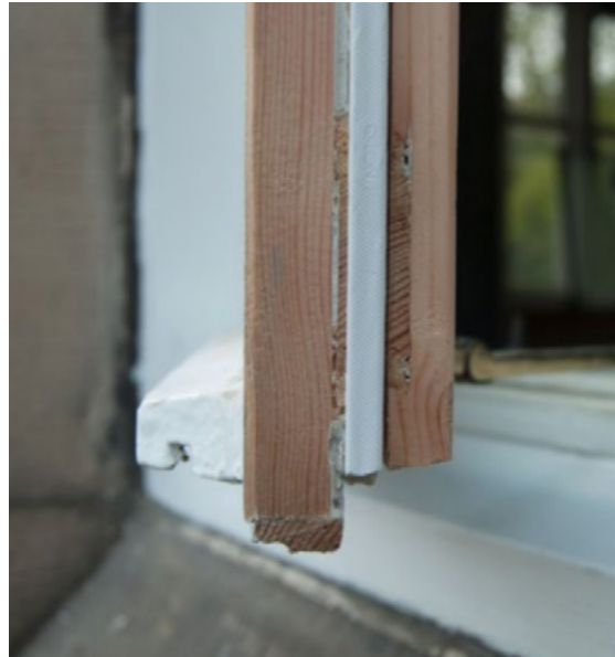
Brush strip on a casement window at Holyrood Park Lodge, Category B listed, LB28023, 11/01/1989, ©Historic Environment Scotland.
