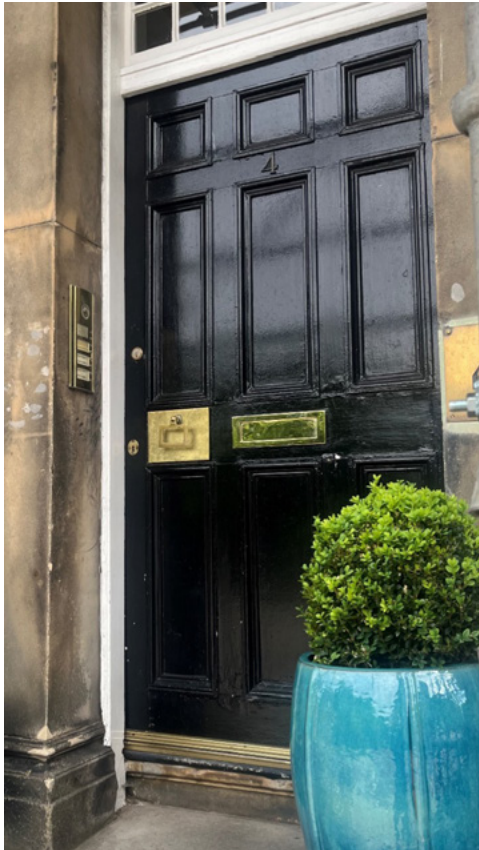
Door Entry system on the door ingoe.
