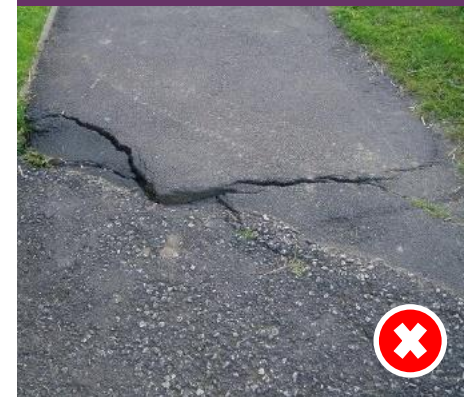
Failed Asphalt Paving
