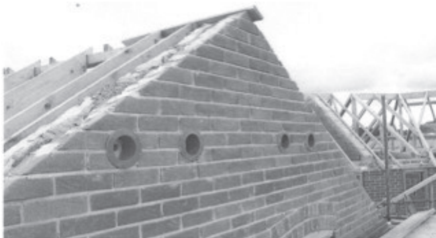
Figure 2 - Swift bricks behind brick work on a new development
